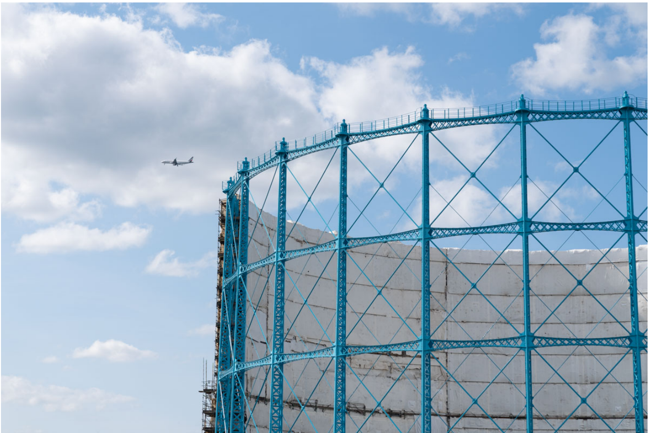
Photographed in July when the scaffolding was still up © Granton Gasometer. 2024 Martin McAdam
