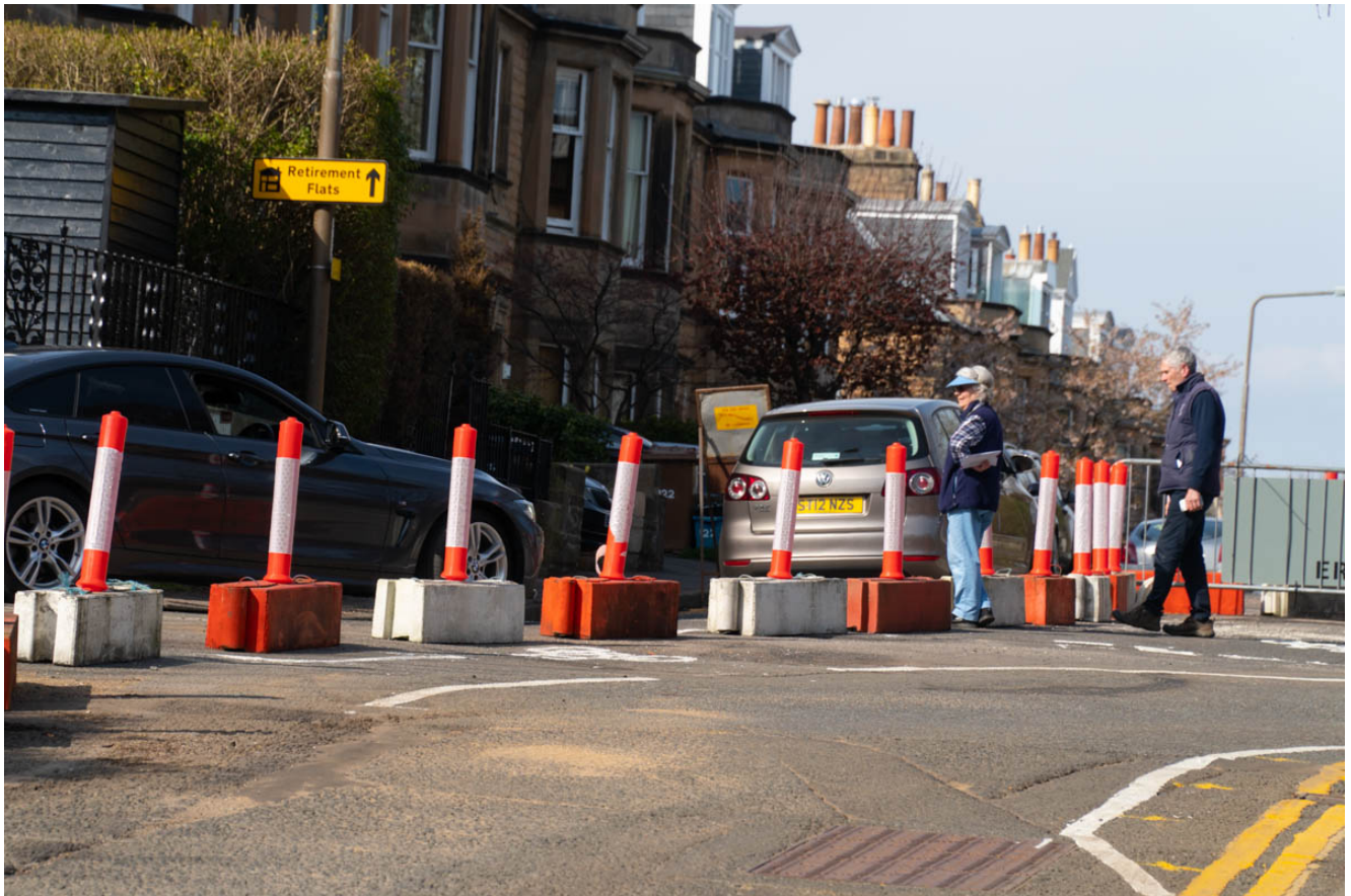
The council made alterations to the layout at Braid Road in anticipation of reopening it to vehicles travelling south on 19 April PHOTO ©2021 The Edinburgh Reporter
