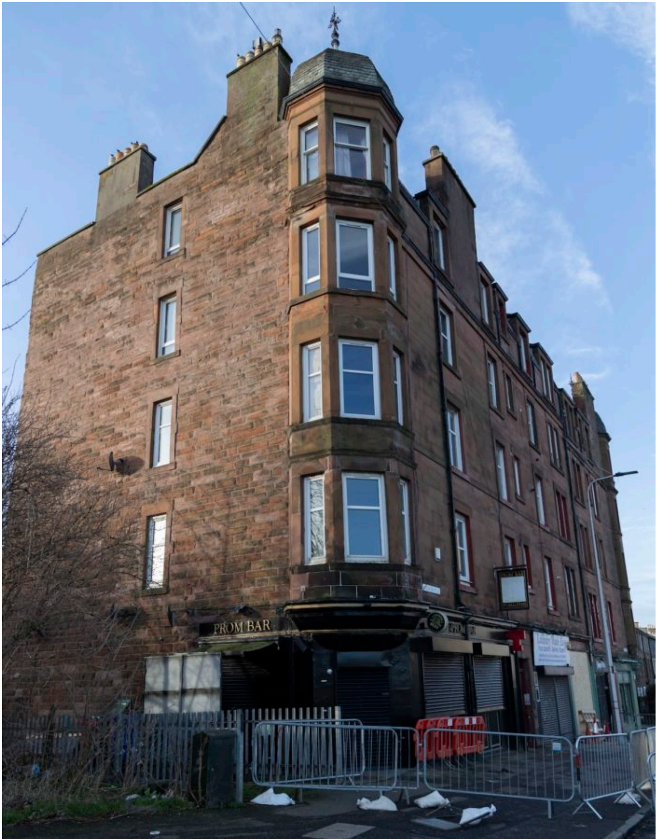
24/1/2024 Picture Alan Simpson Damage to building at Anchorfield near Lindsay Road Edinburgh has made it unsafe.
