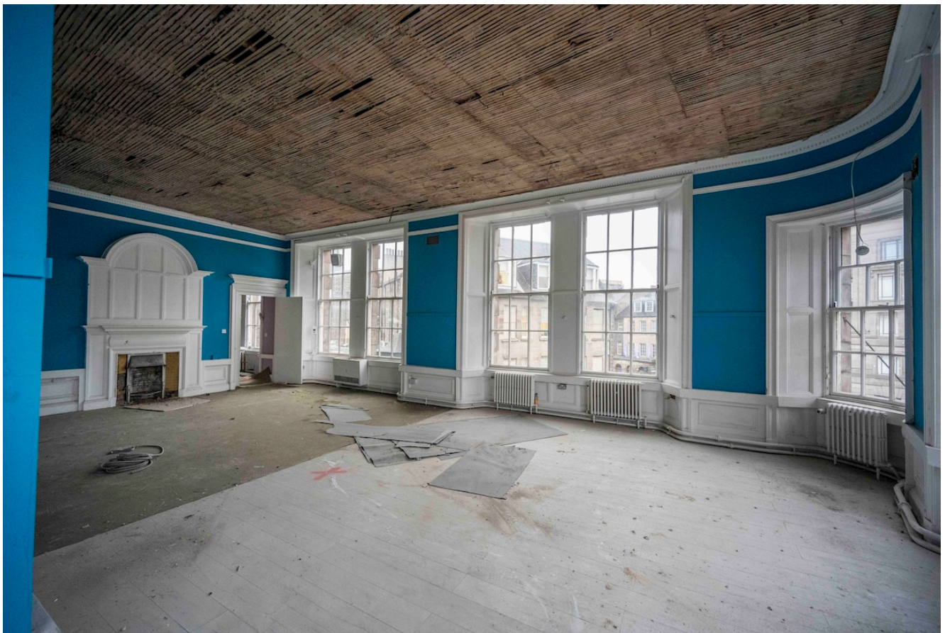
Images of the building in its current state parts of the building have been a hostel and also the Fantasy Loung bar. Picture Phil Wilkinson
