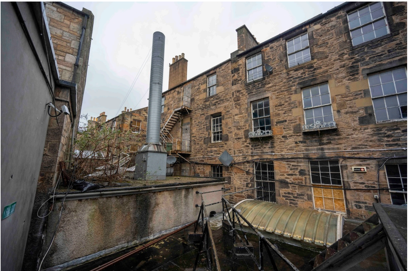
Development of 3 Queensferry Street, Edinburgh, by the Chris Stewart Group. Images of the building in its current state parts of the building have been a hostel and also the Fantasy Lounge bar . Picture Phil Wilkinson
