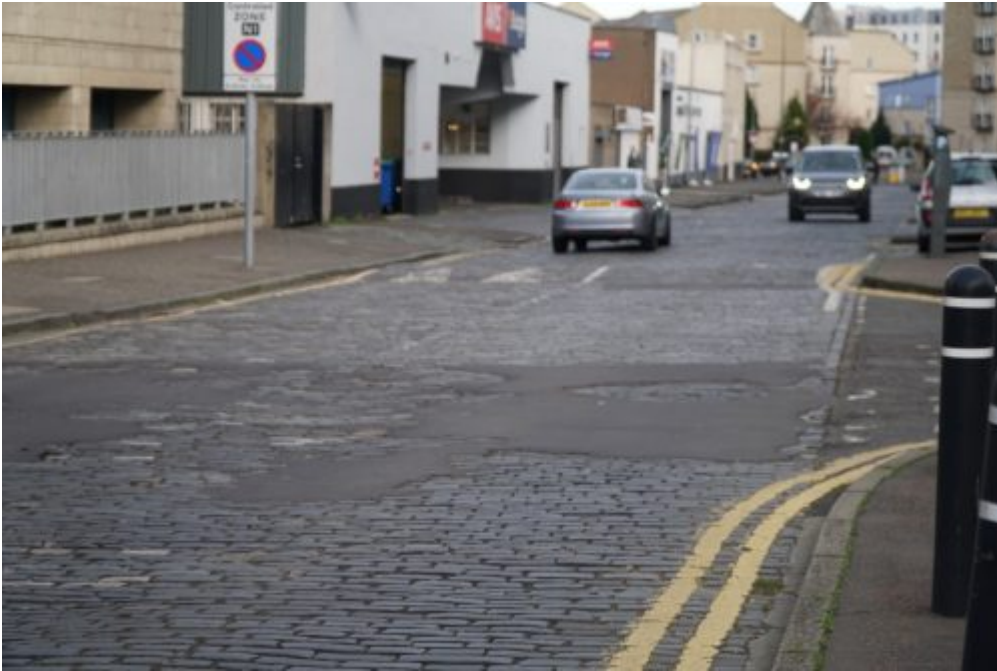
East London Street which residents say has been in a poor state of repair for several years
