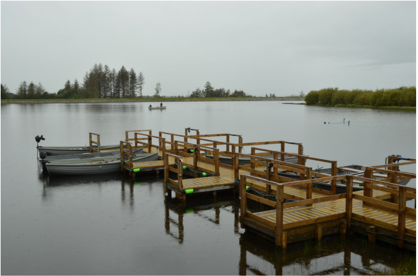
The newly completed boat docking platforms at Morton Fishings. Picture Nigel Duncan
