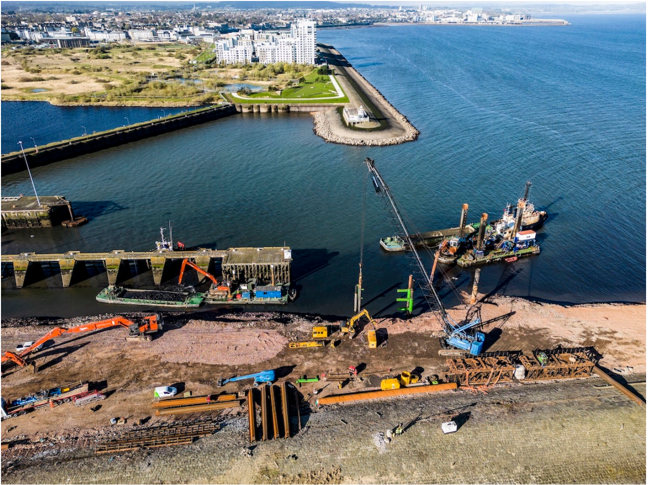
Aerial view of the construction works to create a new riverside berth at Leith Renewables Hub. Pic Peter Devlin
