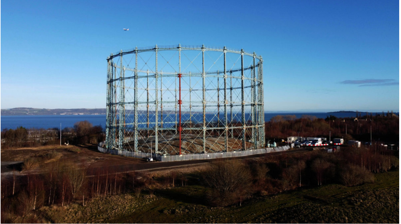
PHOTO Alan Simpson Photography The Granton Gasometer which is being transformed into a new city park.
