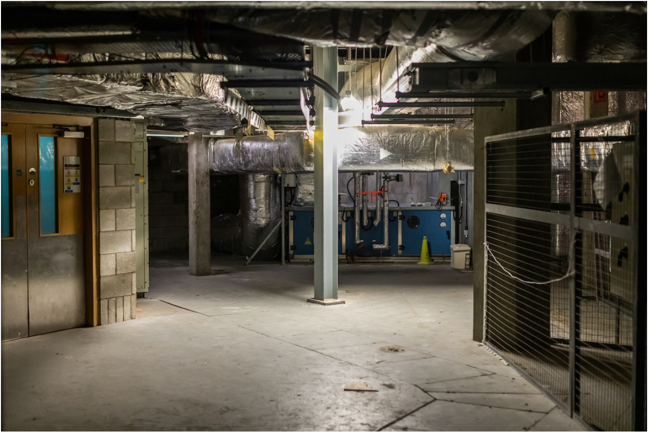
Plant room PHOTO Chris Scott
