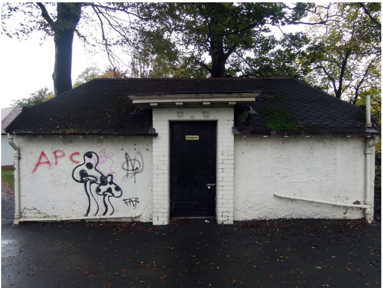
Before the graffiti was removed
