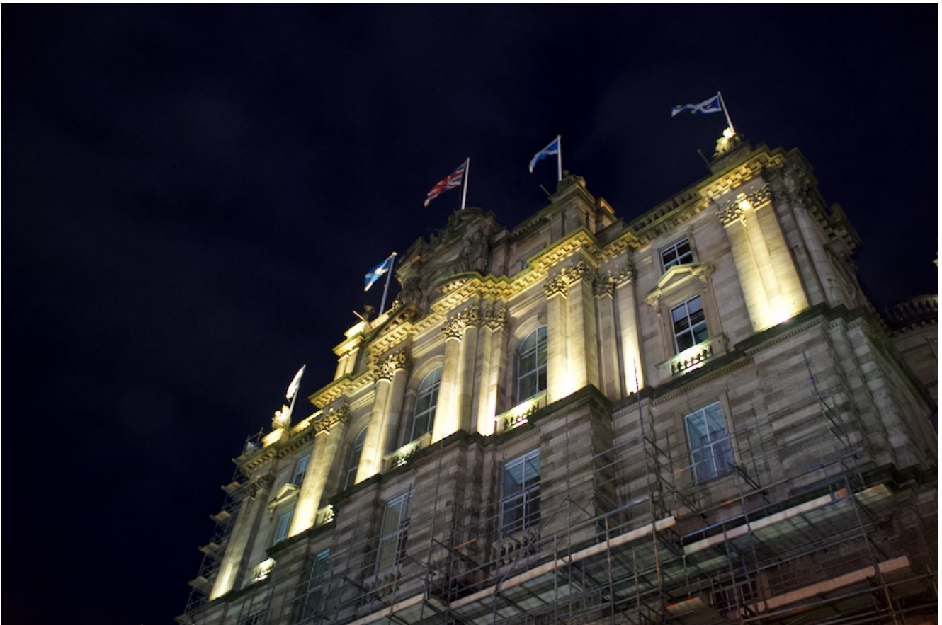
Former Bank of Scotland HQ on The Mound PHOTO ©2020 The Edinburgh Reporter
